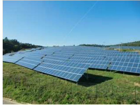
Obr. 12 solární elektrárna (Bor, 09/2011)
